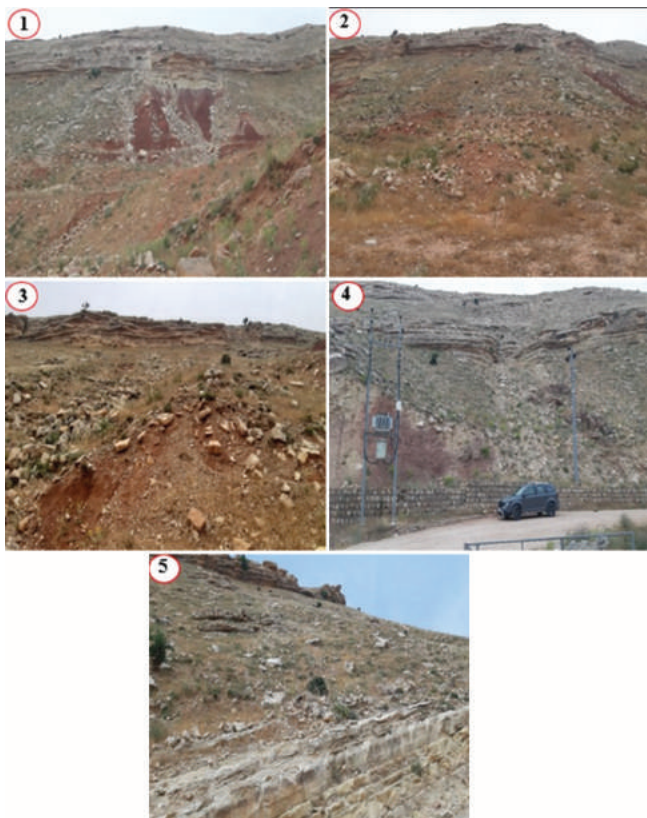
Fig. 6. Right bank station Nos. 1, 2, 3, 4, and 5. Nos. 1 and 4: Active erosion areas indicating unstable slopes. No. 2: Bulged mass in the middle of the slope indicating an unstable slope. No. 3: Recent slid blocks as indicated from the fresh color of the blocks; indicating unstable slope. No. 5: The slope below the cliff is gentler as compared to the other stations; therefore, the amount of slid blocks is smaller and lesser. The reddish brown clastics of the Gercus Formation are overlain by the carbonates of the Pila Spi formation
