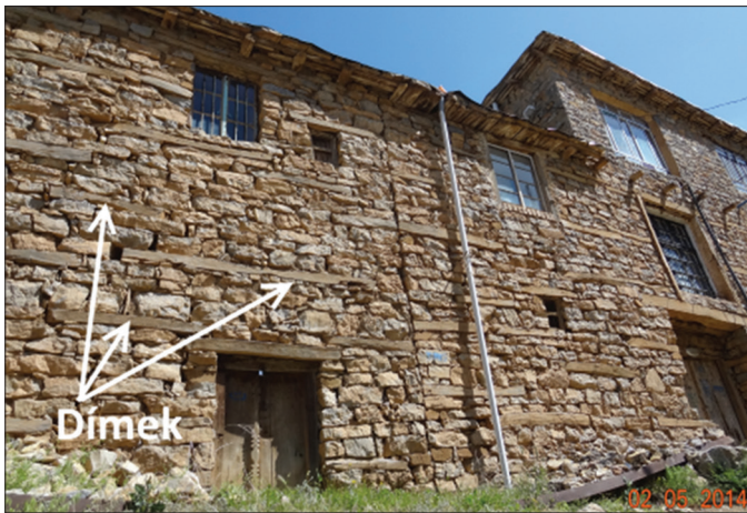
Fig. 8. Positioning Dimek in the stone wall for vertical load distribution as well as withstanding earthquakes. Site visit to the town of Tewélle. (Author, 2014)
