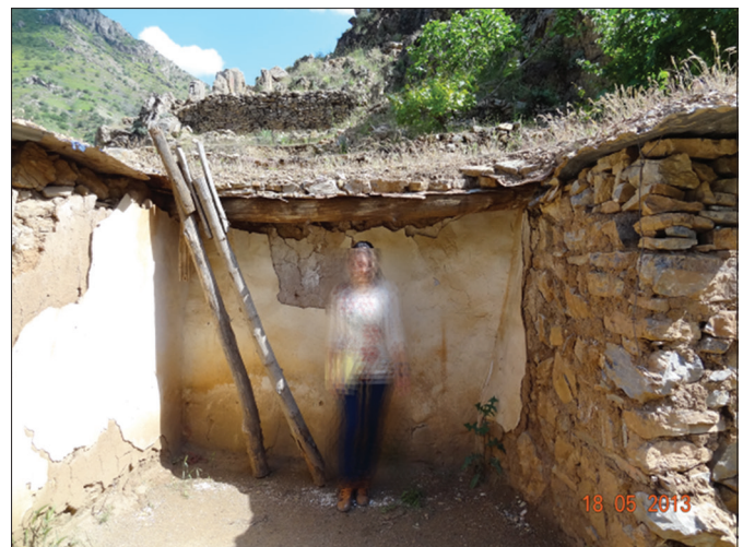
Fig. 14. Height of the ceiling compared with a standing person 1.73 m tall in an abandoned old house in the town of Tewelle. (Author, 2014)
