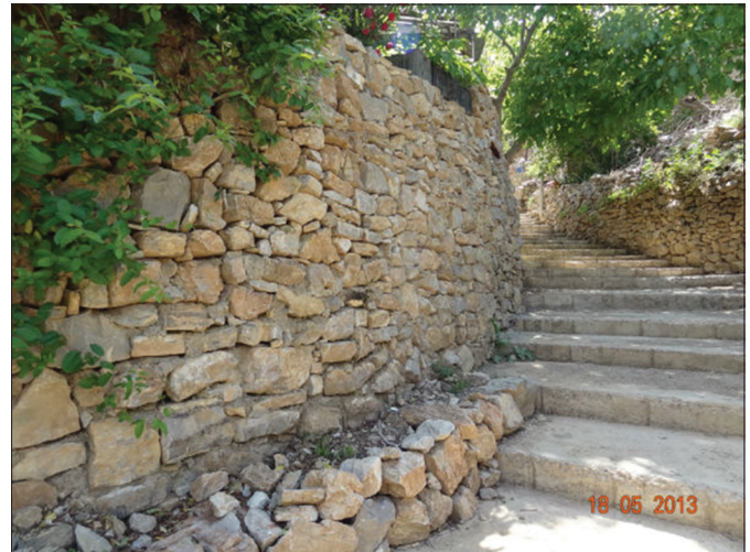
Fig. 10. Alley road to the visited house on the site visit to town of Tewélle. (Author, 2014)
