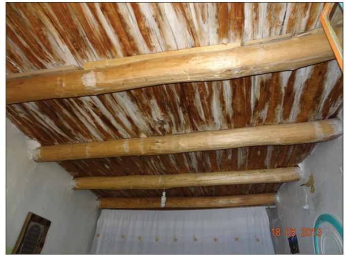
Fig. 17. Roof structure of typical house at the house visited in the town of Tewéllé. (Author, 2013)
